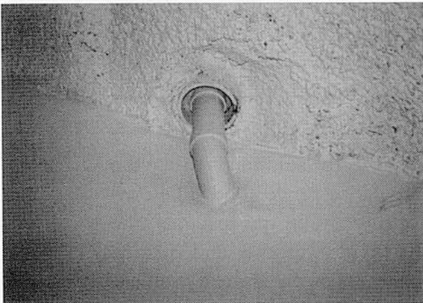
Figure 52a Vent pipe for a bathroom exiting into a utility room.
