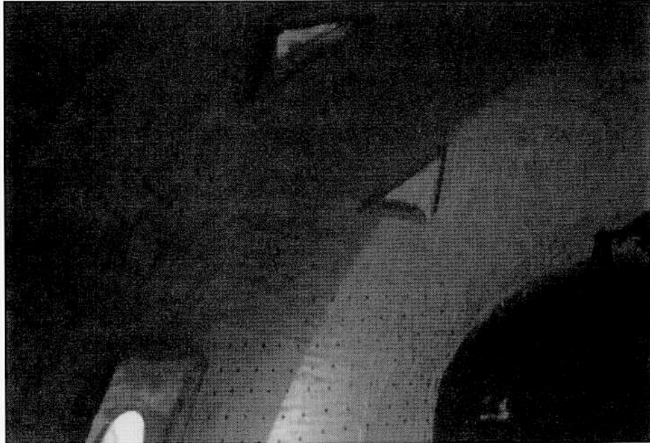
Figure 15 The interior wall and ceiling showing the bucks (frames) for the windows and doors. The dot-like spots are the rebar hangers that have been inserted into the foam.
