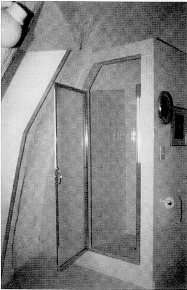
Figure 25 Top of shower door touches the exterior wall but ample room remains for entering shower.
