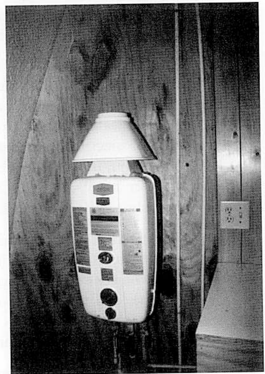
Figure 51 The installed Paloma, water on demand unit.
