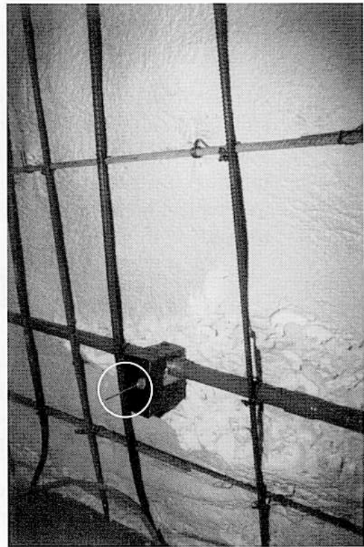
Figure 18 A closer view of the attachment of rebars to the rebar hangers, an electrical conduit and outlet box with the recommended extended tip circled.
